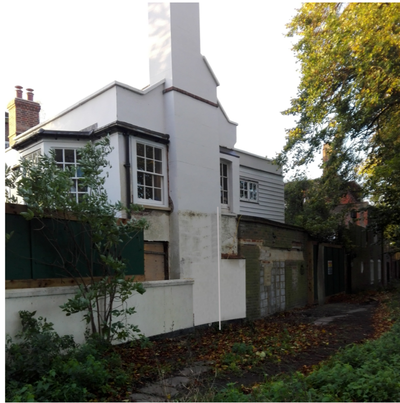
LOCATION A WITH POLE
